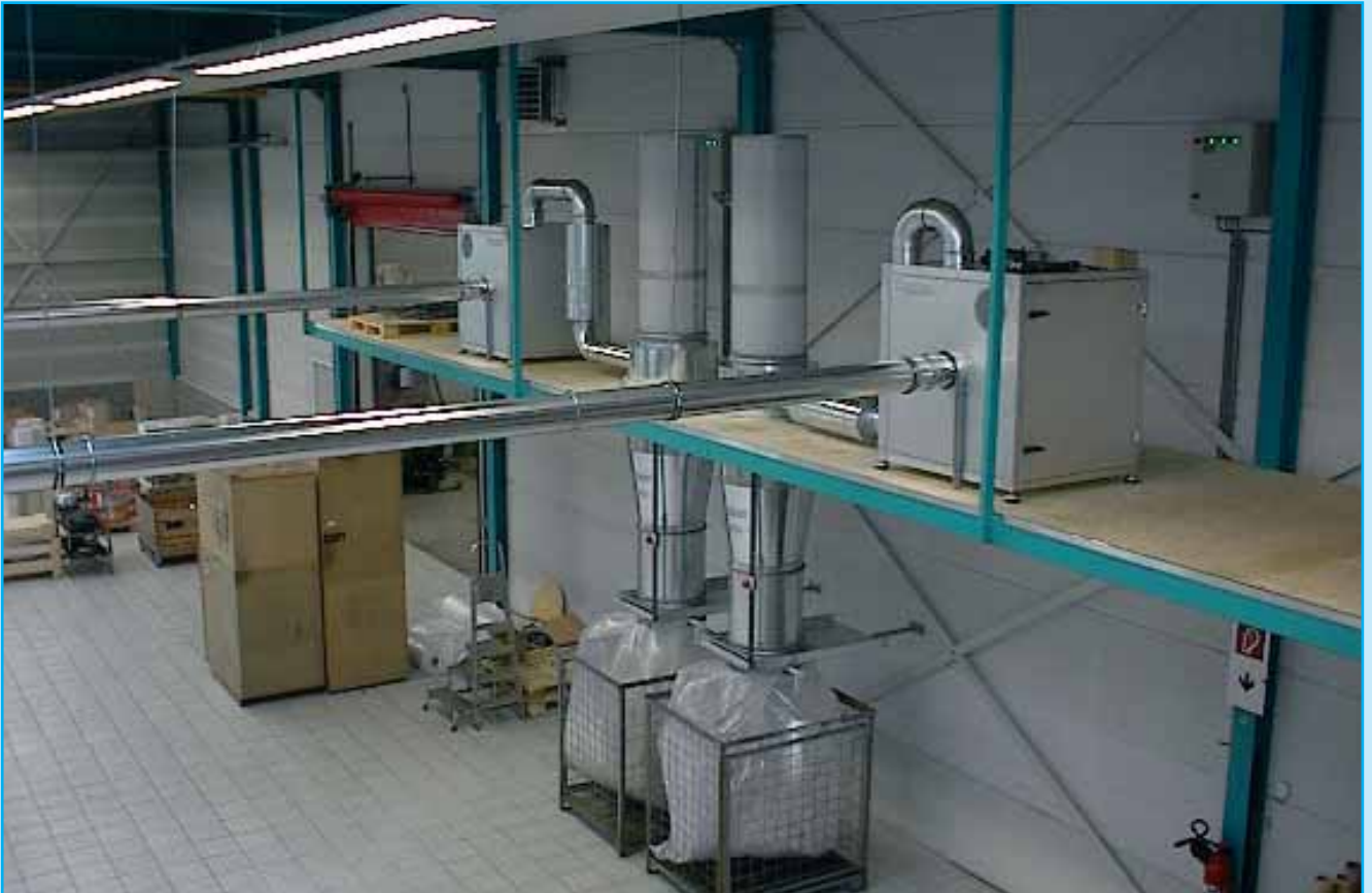
Cyclone systems for collecting two different types of plastic film Each system collects waste from four inspection machines
